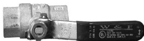
Control Valve "ON"
