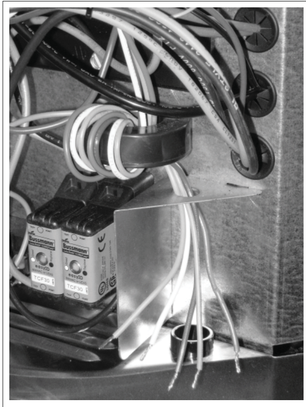
Figure 5. Low Voltage Compartment Control Wiring Connections
