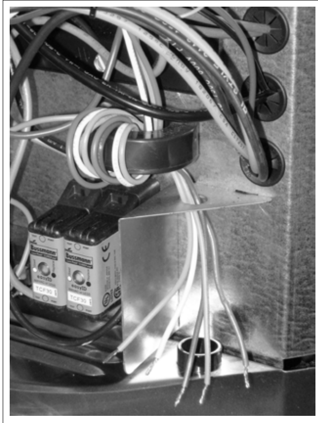
Figure 5. Low Voltage Compartment Control Wiring Connections
