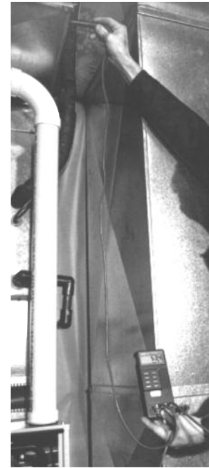
FIGURE 38 TEMPERATURE RISE MEASUREMENT
