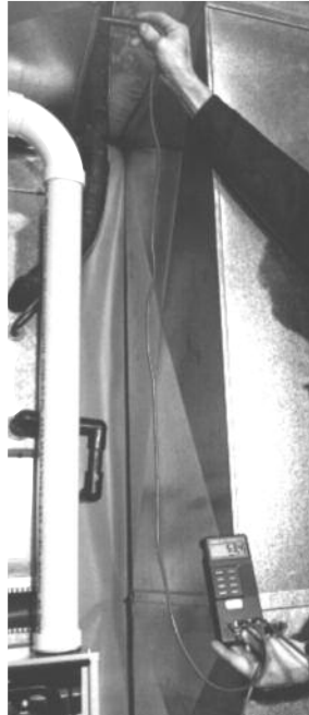
FIGURE 49 TEMPERATURE RISE MEASUREMENT
