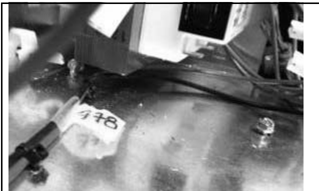
Figure # 26 Primary disconnected
