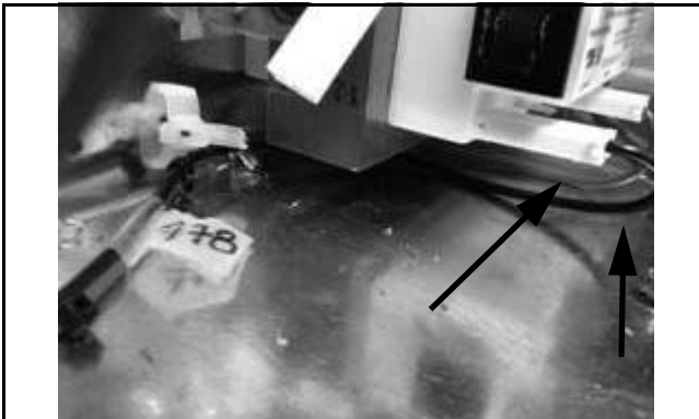
Figure # 25 Transformer primary
